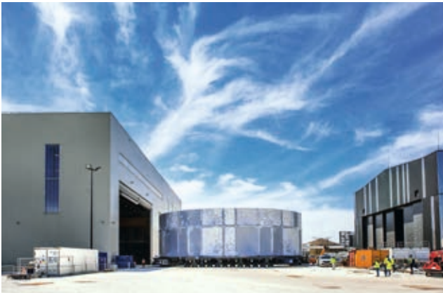
With the assembly of the ITER cryostat - here the “Upper Cylinder” – the Degendorf company once again demonstrates its know-how in complex stainless steel processing.
