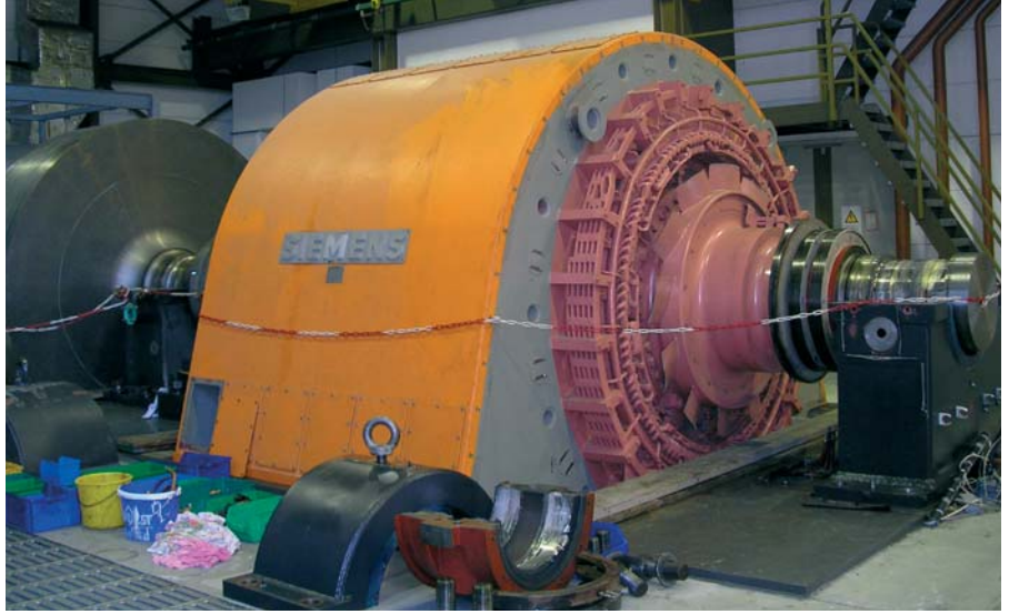
Fig. 1: Damaged flywheel generator EZ4
