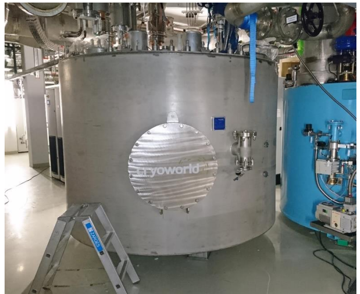
Fig. 2 cryo valve box located in the basement, photo: IPP, B. Kemnitz
