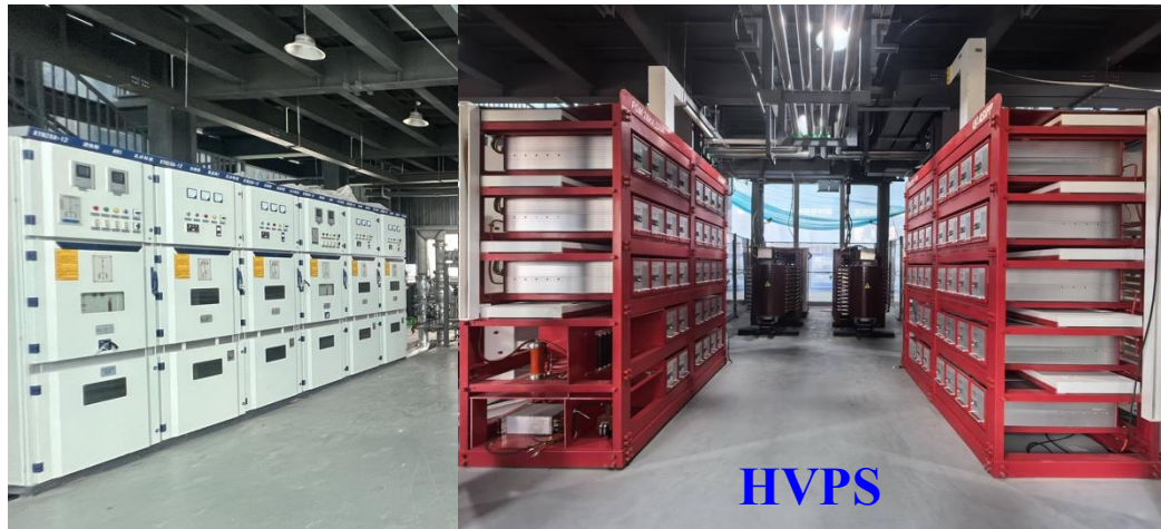
HVPS(10kV, transformer and PSM for transmitter )
