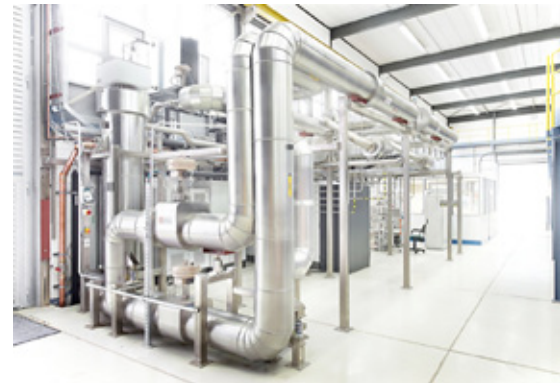
The HELOKA test system at the Karlsruhe Institute for Technology
