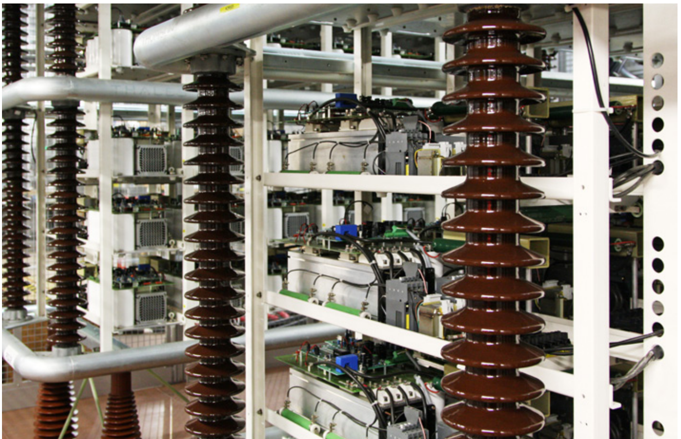
Switching stage racks for the high-voltage DC power system
